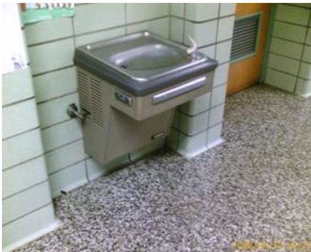
Typical electric water cooler
