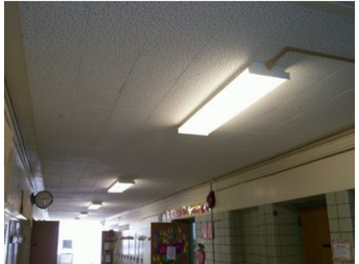
Typical corridor lighting
