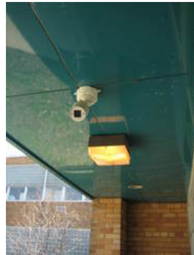
Entrance security camera
