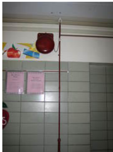
Manual fire alarm bell
