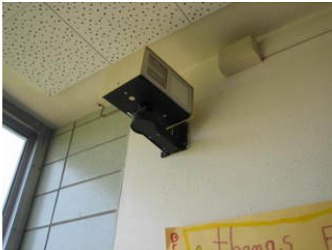
Corridor mounted motion sensor
