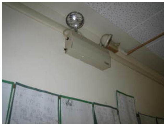
Corridor mounted emergency lighting
