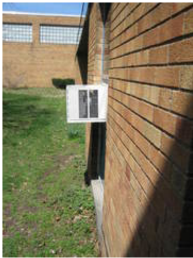
Window air conditioning unit
