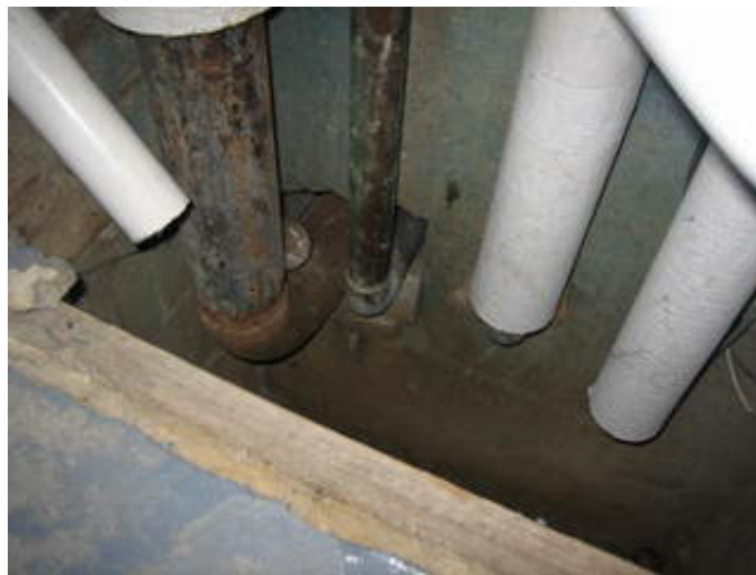
Water service entry
