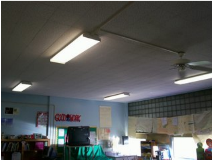
Typical classroom lighting
