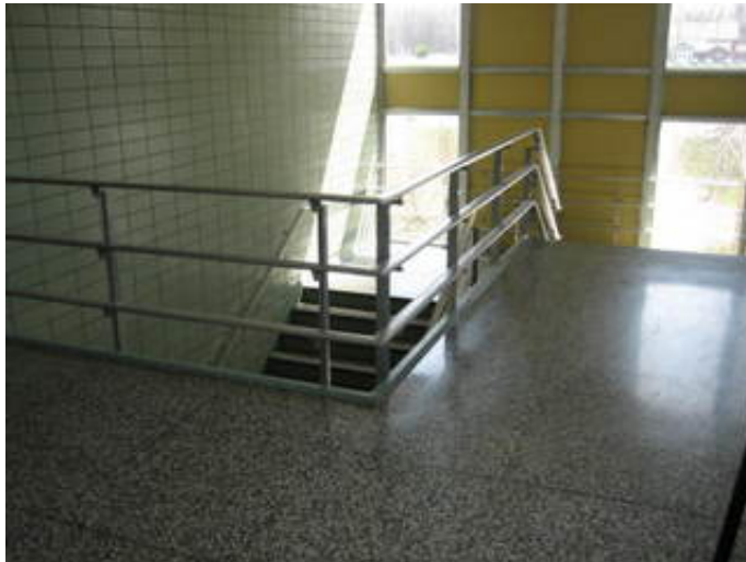
Open stair and non-compliant rails
