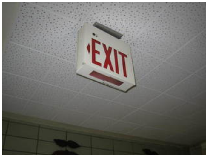
Ceiling mounted exit signage
