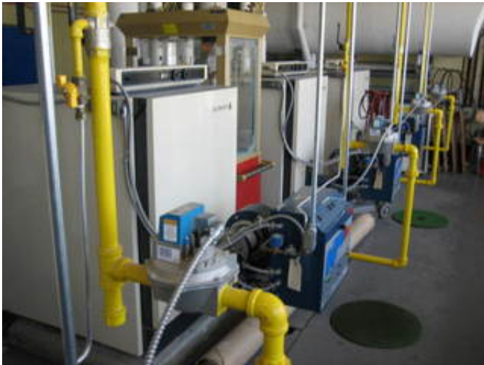
Four (4) hot water boilers
