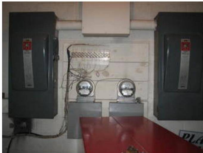
400 amp main disconnects
