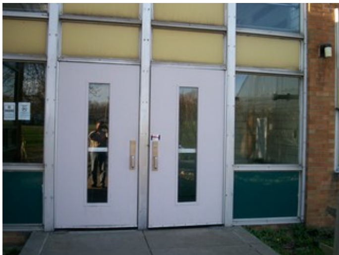
Exterior door system
