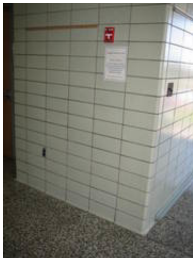
Fire alarm pull mounted high on wall
